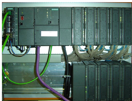
Fig. 4-4: Central PLC – SIEMENS S7-317-2 PN/DP
